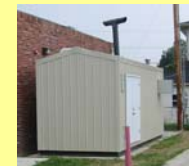
Remediation system equipment building in operation since July 2005
