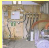
A remediation system located in Warsaw, Indiana
